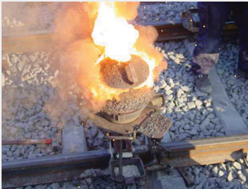
Figure 7.2 “Thermite Reaction.” A small clay pot contains a thermite mixture. It is reacting at high temperature in the photo and will eventually produce molten metal to join the railroad tracks below it.
