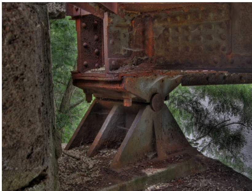
Figure 14.0 “Rust.” These support beams on a bridge are obviously rusted. If the rusting becomes too bad, it will compromise the integrity of the bridge, requiring replacement.
